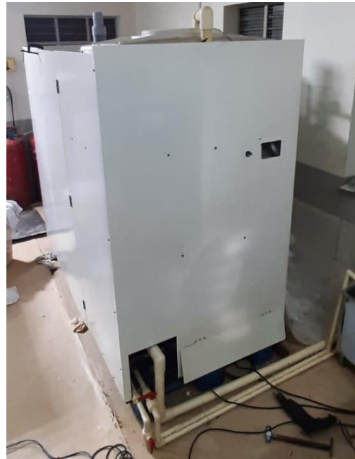
Commercial Laundry ETP
